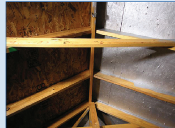
Attic space. The left side does not have radiant barrier and the right side does.
